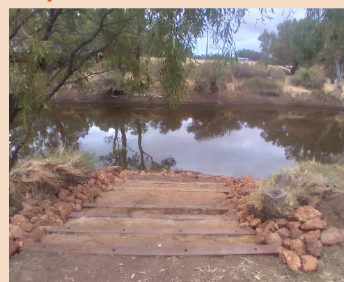
Image: Access steps at Pumphreys Bridge (Works completed by Ben Pike Carpentry)
