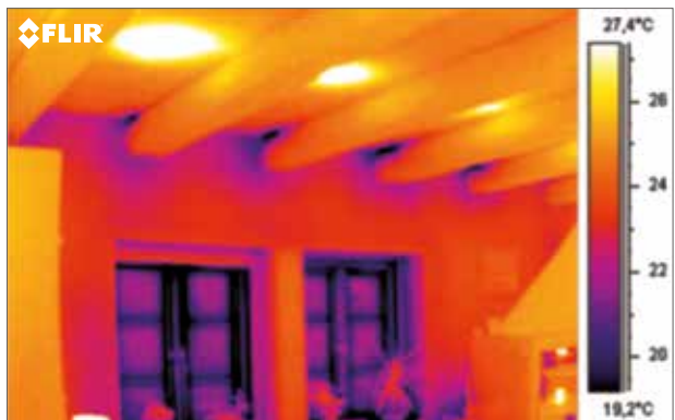
The thermal image shows thermal bridges between the roof beams and adjacent walls.
